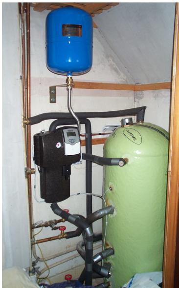
A typical internal installation
