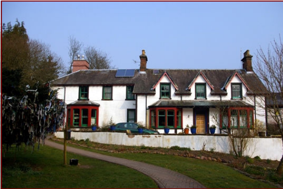
The Solar panels on Johnstone House. Two more systems are in the 'valley' beyond the front roof ridge.
