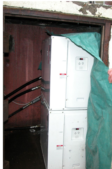
The two 12kW heatpumps in situ
