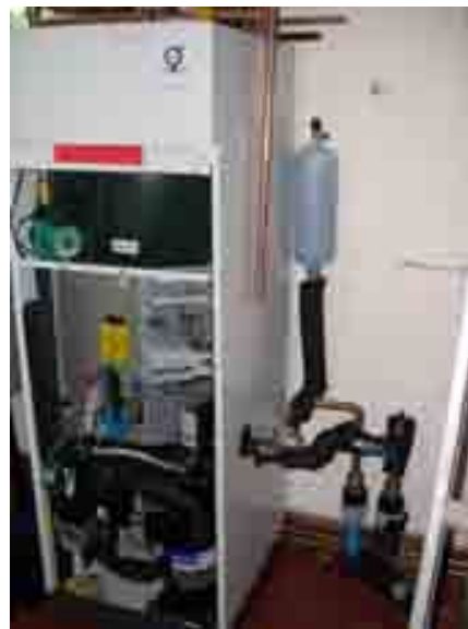
Inside the heatpump, showing the 150ltr tank, the expansion vessel and flow and return pipes from the manhole (not yet fully lagged).
