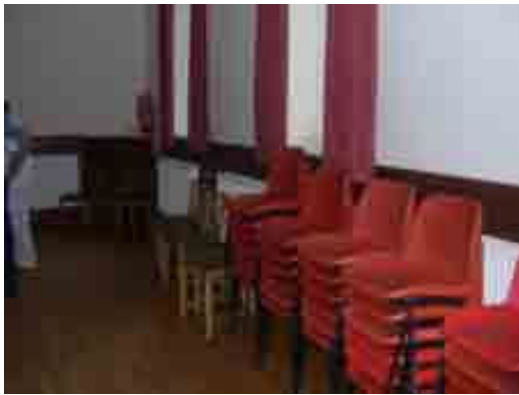
Radiators in the main hall
