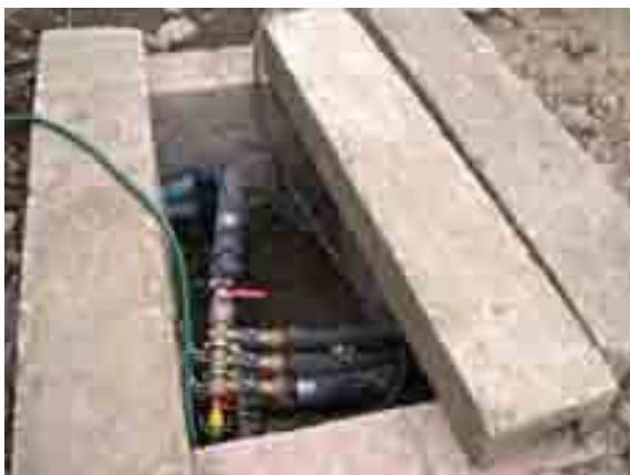
Manhole behind hall with header with flow and return to the three ground loops
